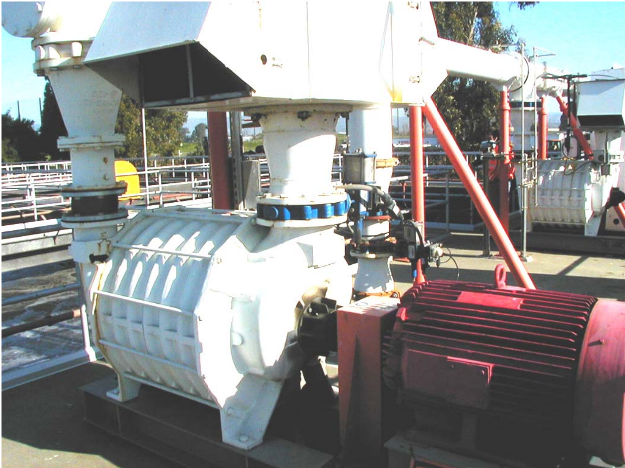
Figure 2.1.1.1 – San Leandro Multistage Aeration Blowers
